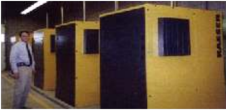
Steve Owen from PERC reviews the finalized installation of six FB 620 100 hp Omega-paKs.
